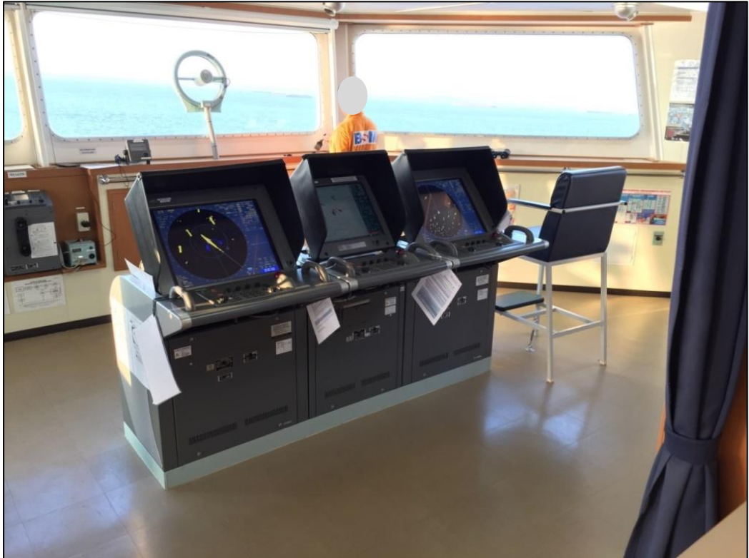
Figure 4: Radar sets and ECDIS located on the starboard side
